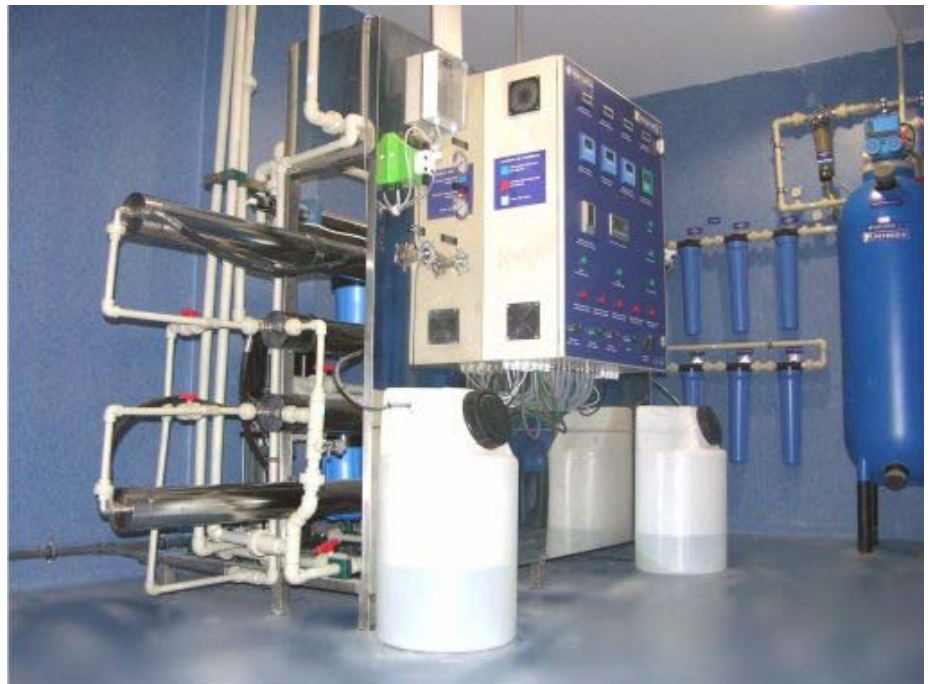
Photo: Petsea Ro-TWH Installation in Meixoeiro's Hospital (Vigo).
