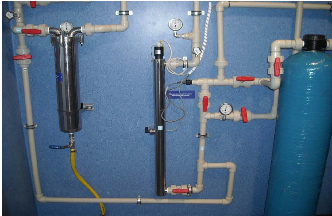
Photo: Ultraviolet sterilizers installation.
