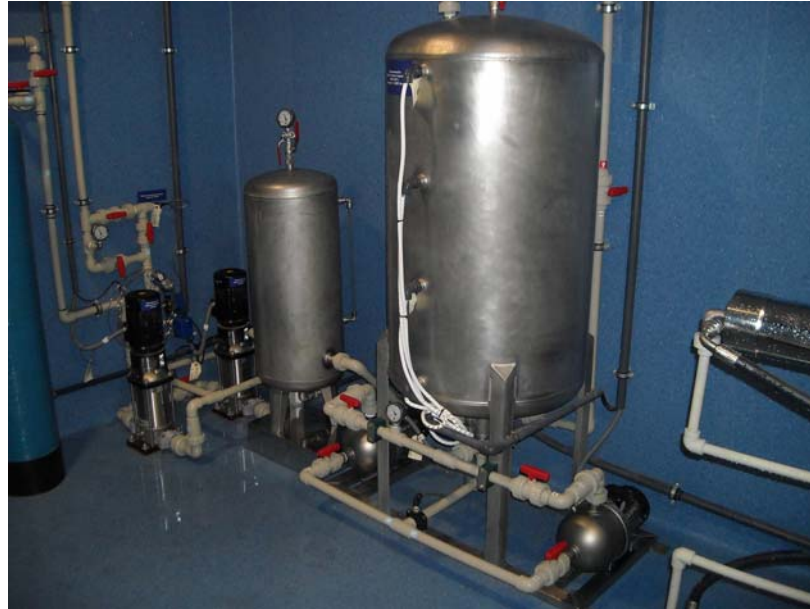
Photo:Flector tank, pumping group and storage prior to ring.
